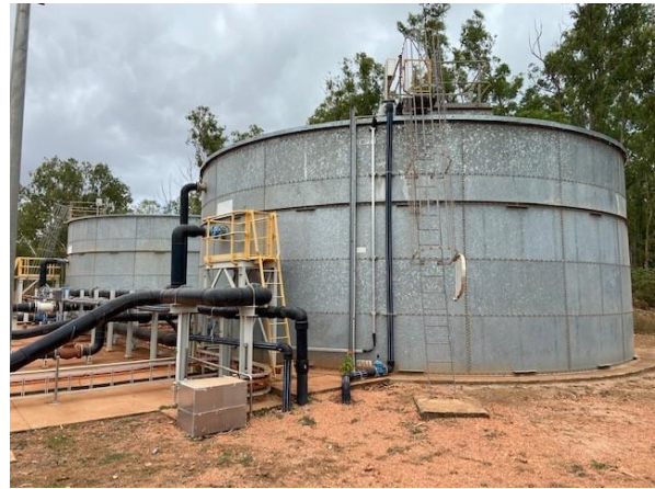
Figure 3-10 Evans Landing Potable Water Tanks
