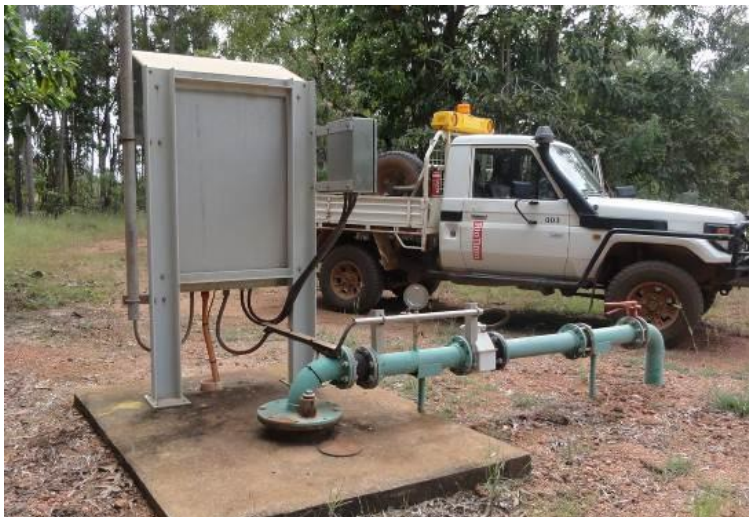
Figure 3-7 Typical Borehead located on RT Weipa Site (SA12)
