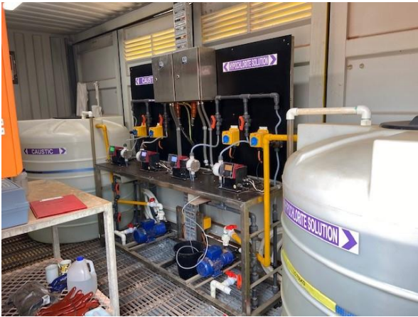
Figure 3-9 Evans Landing Dosing Systems
