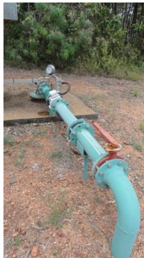
Figure 3-8 Typical Borehead located on RT Weipa Site (SA12)
