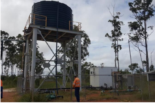
Figure 3-13 Elevated Storage Tank
