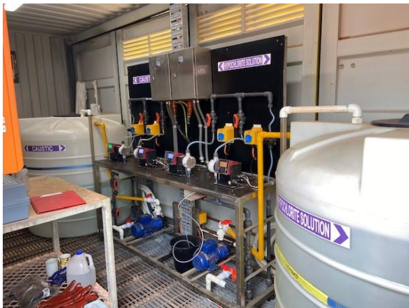
Figure 3-9 Evans Landing Dosing Systems
