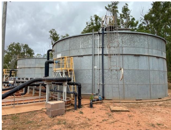
Figure 3-10 Evans Landing Potable Water Tanks
