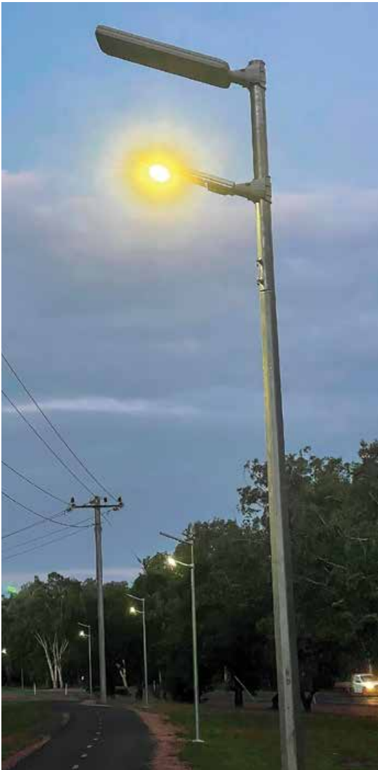
Central Avenue pathway solar lights
