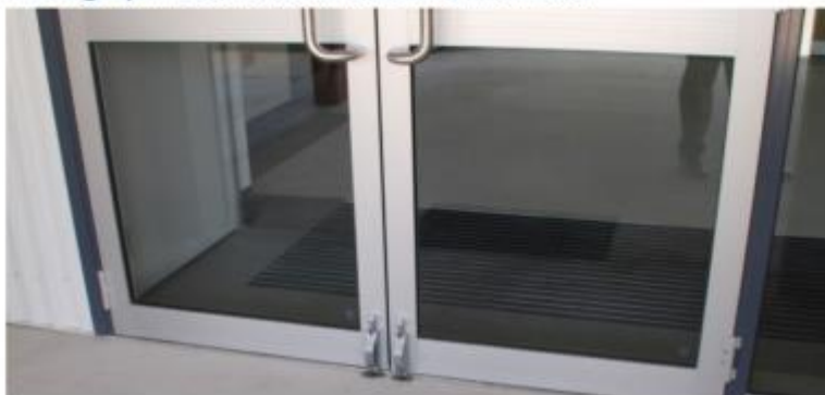
Photograph: Lock bolts on bottom of front door
