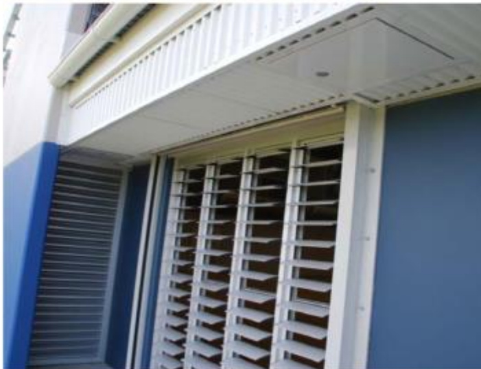
Photograph: Roller shutter control access panel
