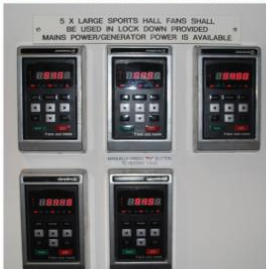
Photograph: Controls to sports hall ceiling fans
