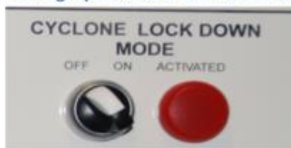
Photograph: Shelter ventilation lock down switch
