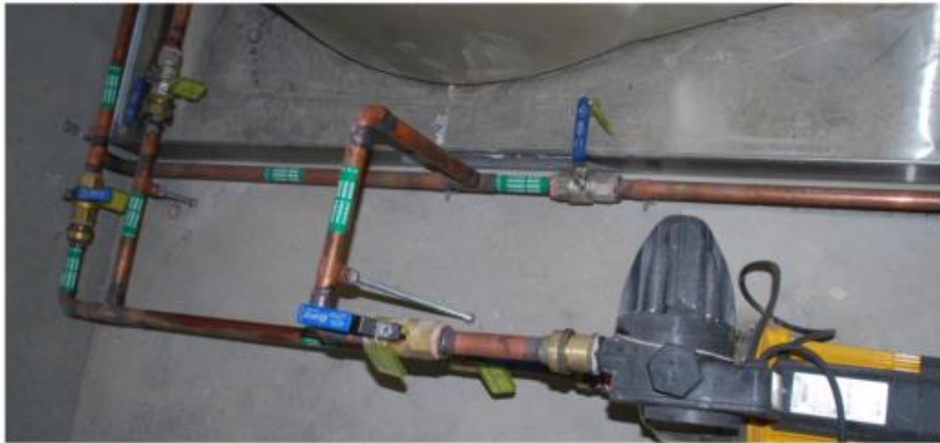
Photograph: 5kL tank pump and valves
