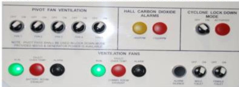
Photograph: Pivot fan, battery room, comms room & toilet controls and alarms
