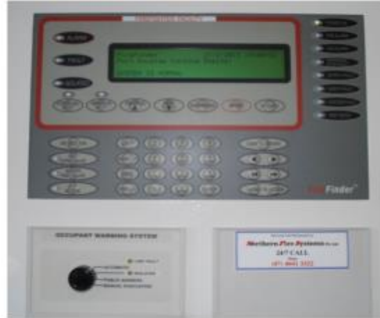
Photograph: View inside board
