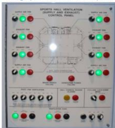
Photograph: Ventilation control panel
