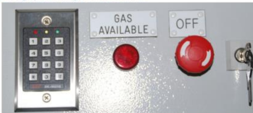
Photograph: Master gas control in kitchen
