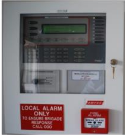
Photograph: Fire control board
