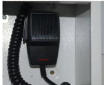
Photograph: Emergency public address microphone
