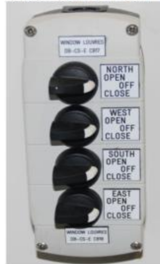
Photograph: Close upper level panels with controls in staff room
