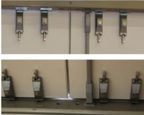
Photograph: Lockbolts on sports hall doors
